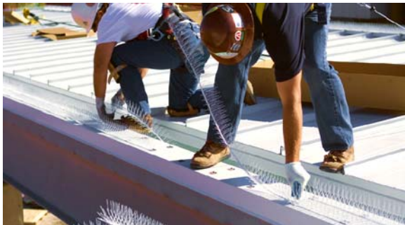
More than 45,000 feet of Premium Nixalite in three different ColorCoat colors were installed on the 4th Street Station.
